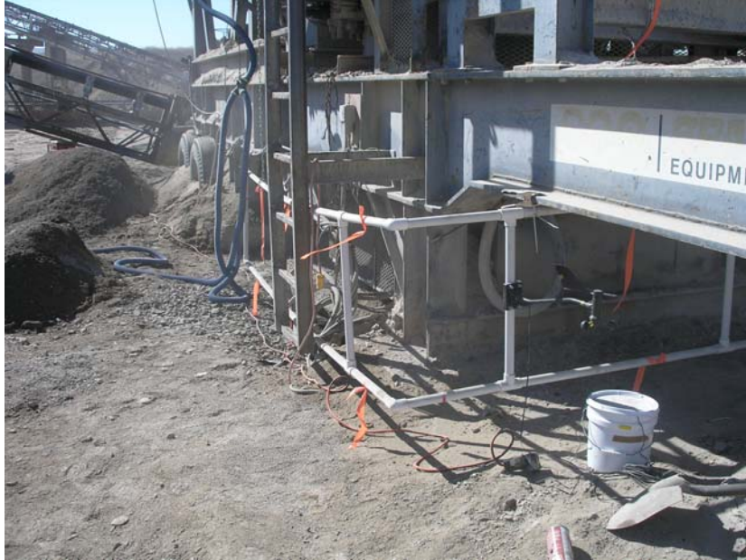
Figure 2-8. Close-up Side View of Crusher Lower Array, Barstow Transfer Point
