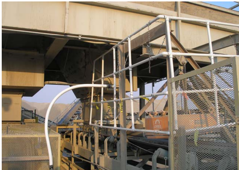
Figure 2-28. Conveyor Transfer Point Array, Vernalis
