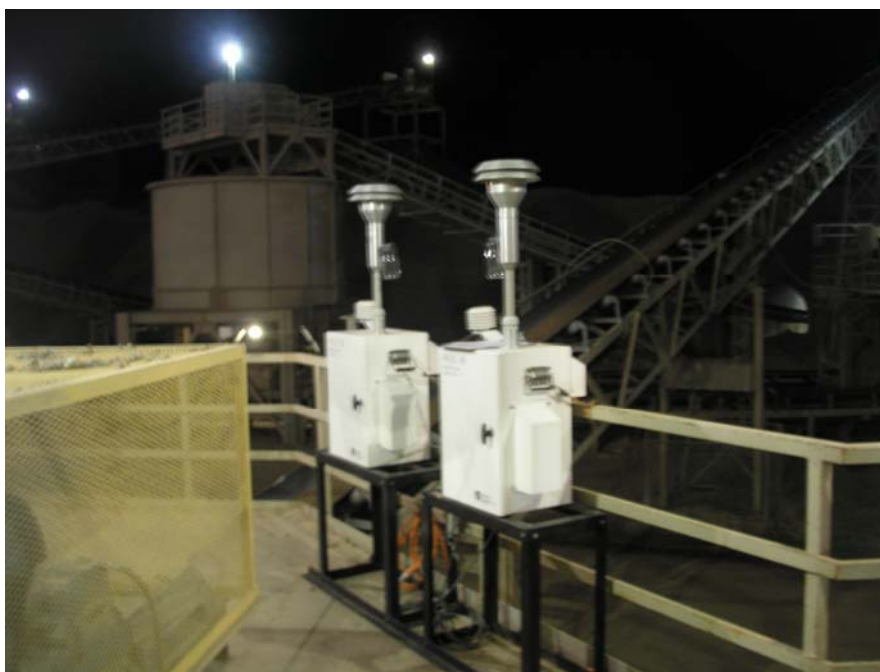
Figure 2-30. Process Equipment Upwind Monitors for Screen and Transfer Point Tests, Vernalis
