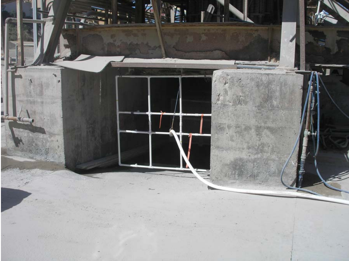
Figure 2-17. Side View of Crusher Discharge Array, Carroll Canyon
