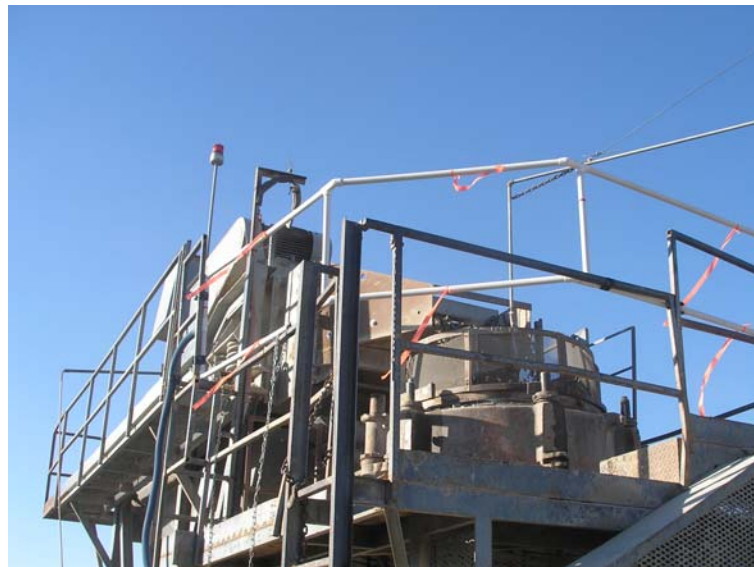
Figure 2-7. Side View of Upper Crusher Array, Barstow
