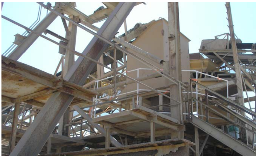
Figure 2-16. View of Crusher Inlet Sampling Array, Carroll Canyon
