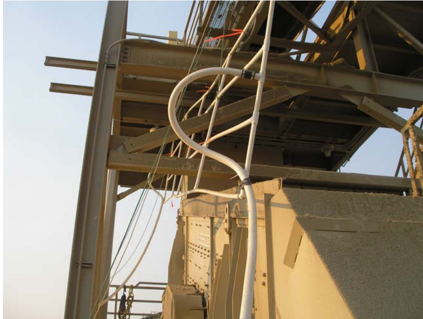
Figure 2-25. Side View of Vibrating Screen, Vernalis
