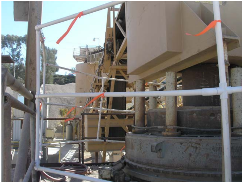
Figure 2-15. Side View of Crusher Inlet Sampling Array, Carroll Canyon
