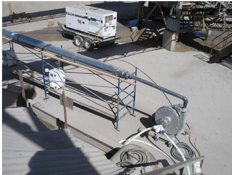
Figure 2-3. View of Centrifugal Blower and Combined Sampling Duct, Carroll Canyon (FRM 2000 PM 4 Monitor Center-Left, PM 10 TEOM Left)
